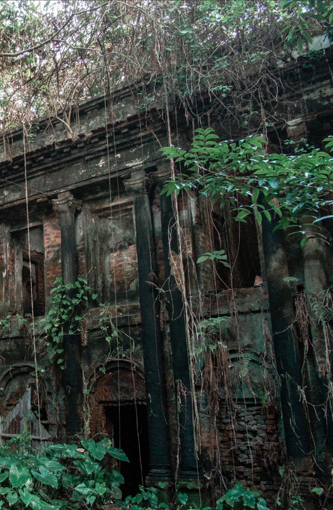
The decaying remains of an abandoned Jamidar house lie in deep isolation. Photograph by Nahid Hasan. 2020.
