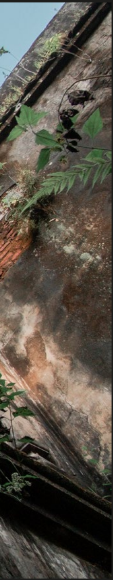
Top left: The fading outlines of an abandoned Jamidar house can be seen as its cracked walls slowly erode and wild plants and creeping branches grow over the structure.
