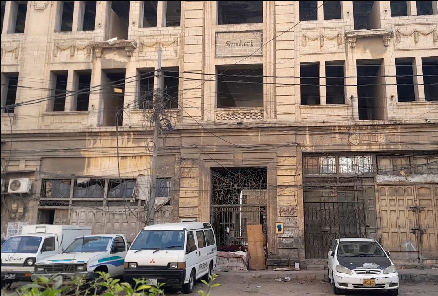
The Sevakunj Building, originally a student hostel offering indoor ventilation, now sits abandoned Photography by Wara Irfan
